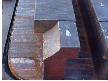
Failure of Tee head attachment in field pole of pumped storage generator. Figure 4.
