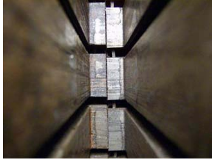
Stator Core Displacement at core split and bottom of coil slot. Figure 8.
