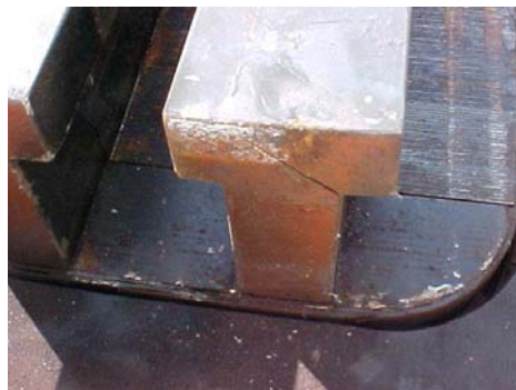
Crack in Tee head field pole attachment on pumped storage generator with many starts. Figure 3.
