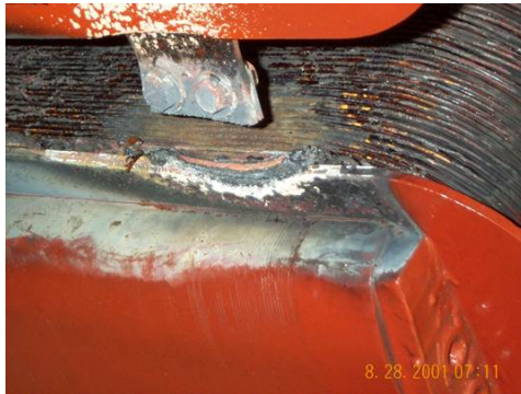
Cracked and failed pole to pole connector. Bolted and soldered solid cross section. Figure 2.
